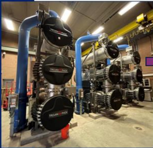
Advanced Oxidation Process (AOP) Ultraviolet (UV) light with injected hydrogen peroxide create a strong oxidant that removes 1,4-dioxane and trichloroethene from water.
